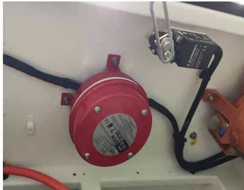
Figure 5-36 Aerosols activated by thermal sensitive wires
